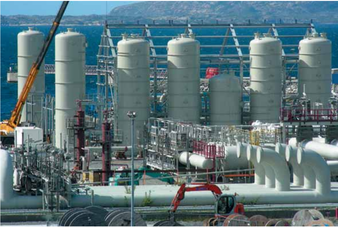
Mongstad's vapour recovery plant. Source: Aker Kvaerner Cool Sorption
